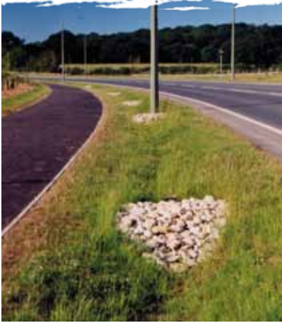
Witney, Oxfordshire – a stone check-dam in a roadside swale to slow flows and prevent erosion. Stones that become hidden in grass may pose management risks. Photo: Bob Bray
