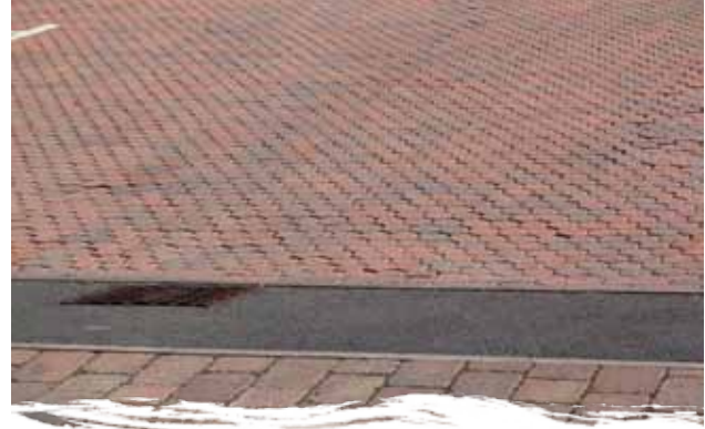
Fort Royal Primary School, Worcester – block paving is one of a number of permeable surface types facilitating water filtration into the ground below or collection chamber. Photo: Bob Bray
